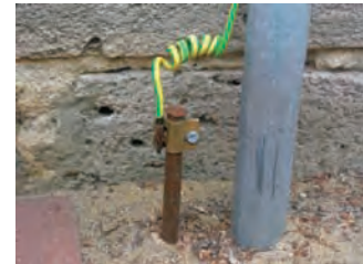
A typical earthing electrode (left of gray pipe), consisting of a conductive rod driven into the ground.
